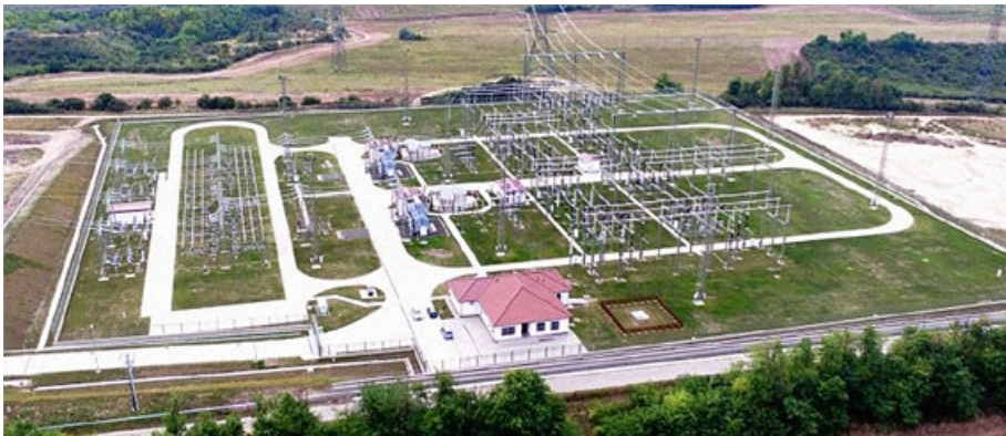
Figure 7: MAVIR ZRt. Kerepes 400/120 kV substation. Source: (URL8)
