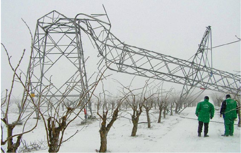
Figure 5: Falling post on a 220 kV dual-system transmission line. Source: (URL6)
