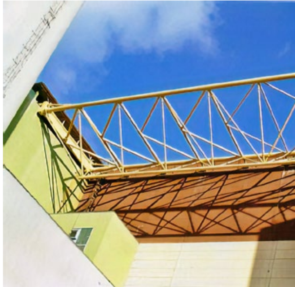
Figure 6: Paks Nuclear Power Plant Earthquake Reinforcement Brace Steel Bridge Structure Between Localization Towers. Source: (URL7)
